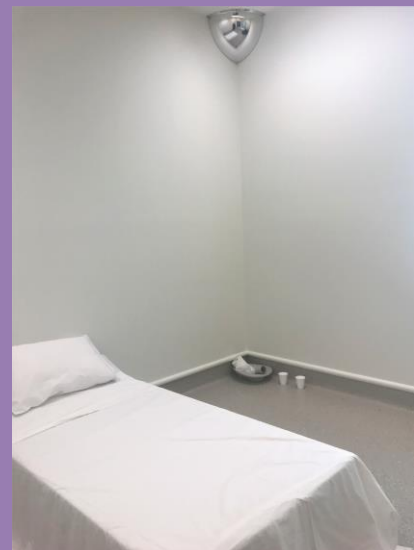
Seclusion room from a regional Victorian hospital Image supplied under the condition the source remains anonymous
